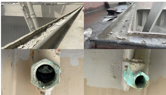
FIGURE 5 Hardened cement in drain channels and drain holes
