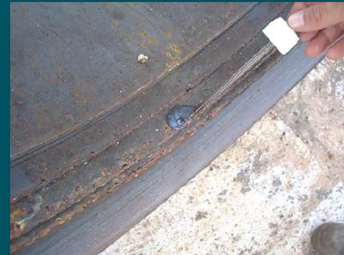
A positive result using the silver nitrate test on rust areas of a telescoping HRC: will require lab verification
