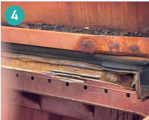
Figure 4: Drain channels on cross joints and coamings should be free of debris. Rubber packing should be in good order to help with the weathertight integrity of the hatch covers.
