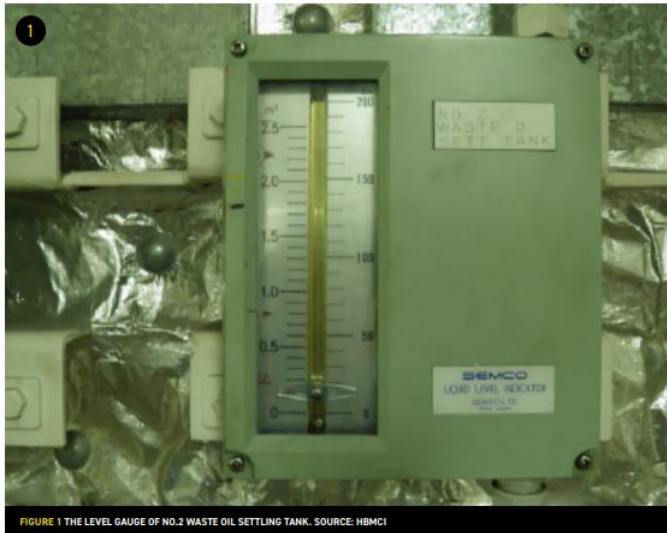
FIGURE 1 THE LEVEL GAUGE OF NO.2 WASTE OIL SETTling TANK. SOURCE: HBMCI
