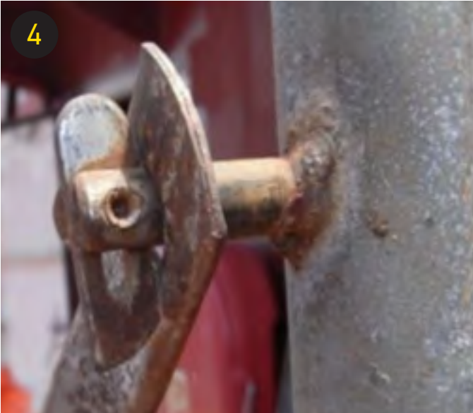
FIGURE 4 LOOSE SCAFFOLDING CROSS BRACE LOCKING PINS ALLOWING TRAVEL UP TO 40 MM. SOURCE: AUSTRALIAN TRANSPORT SAFETY BUREAU (ATSB)
