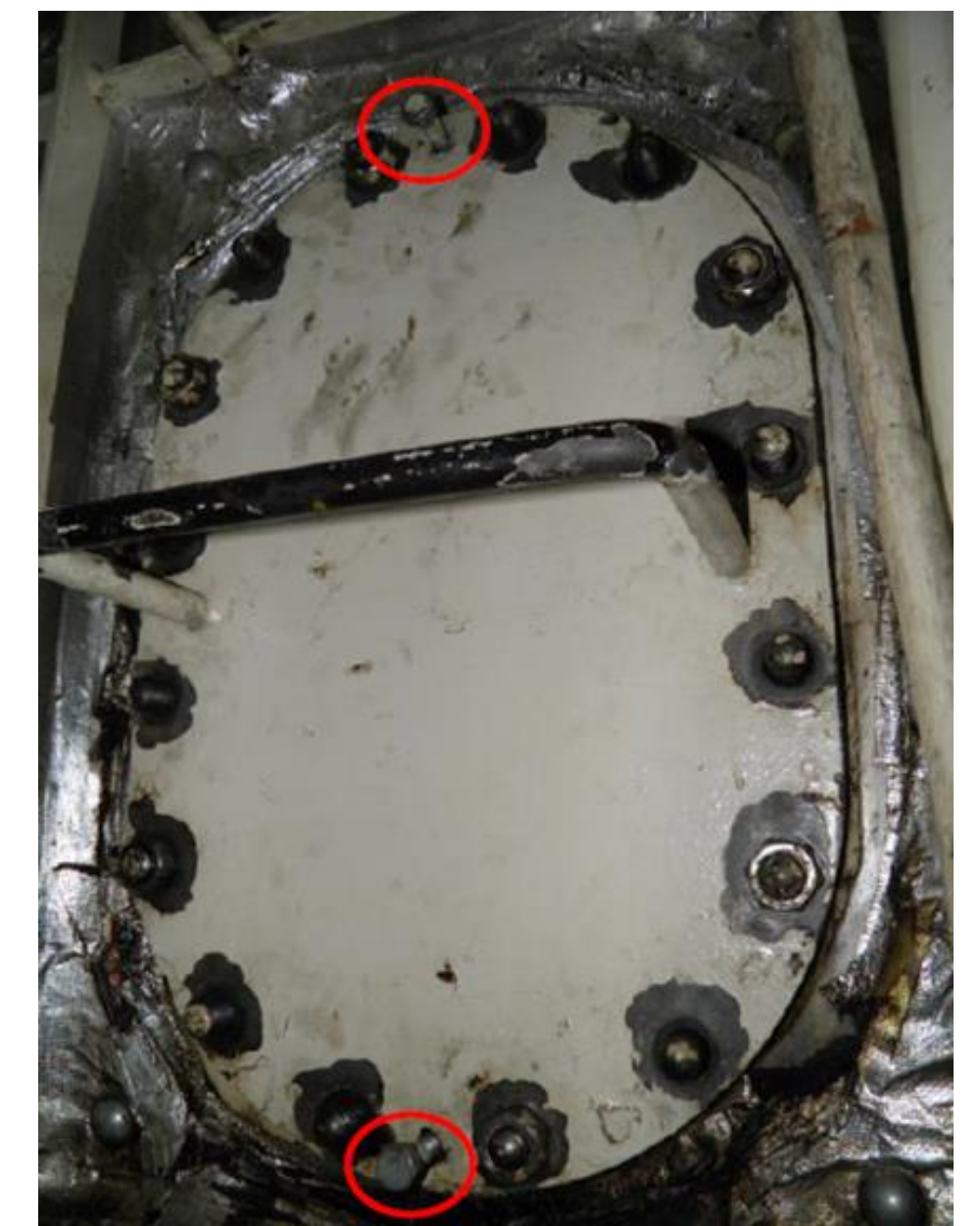
The manhole cover of the tank and the two jackscrews fitted on the top and bottom side. Source: HBMCI
