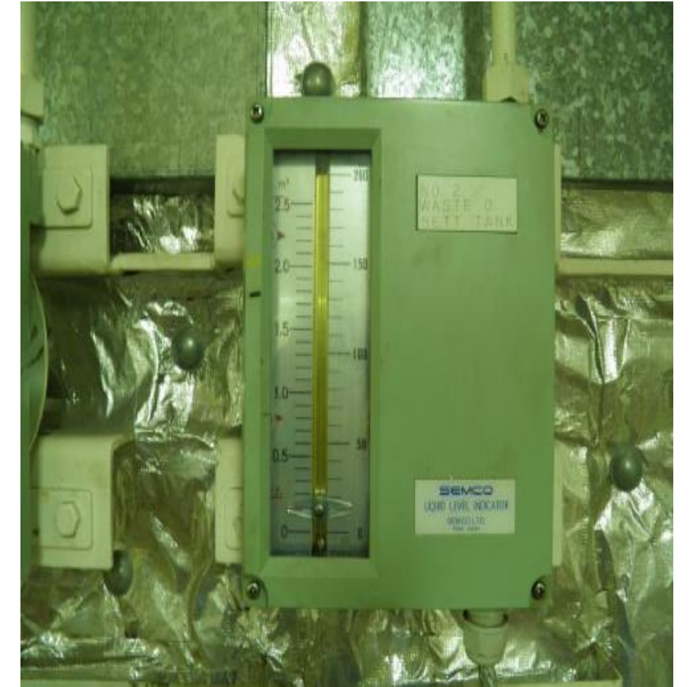
The malfunctioning level gauge
