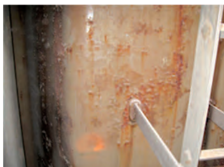
Deterioration of tank coating.
