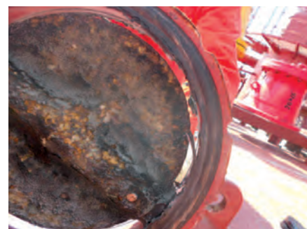
Damaged drop valve.
