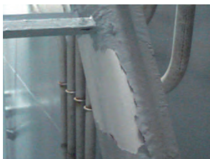
Tank coating damaged due to excessive heat.
