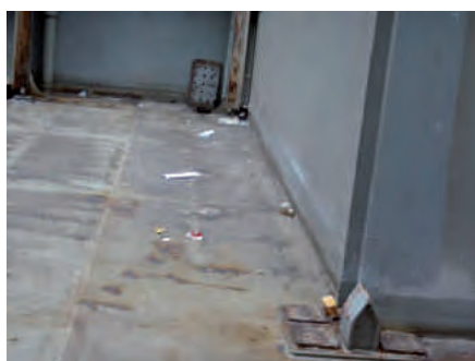
Rubbish on tank top plating
