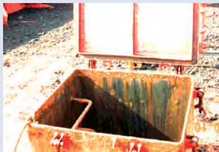
Evidence of water ingress at the cargo hold entrance hatch and the hatch coaming.
