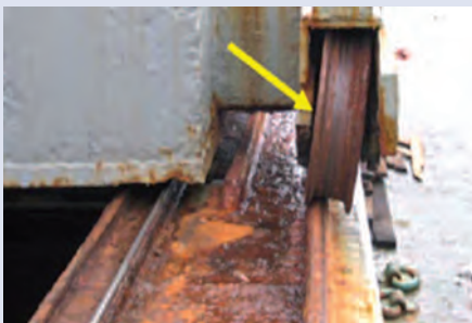
Hatch cover guide wheel bearing failed – hatch cover will not close evenly.
