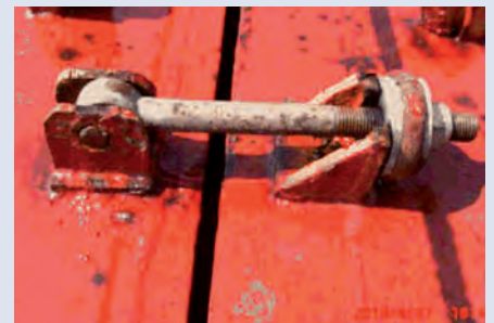
Cross joint cleat renewed but old perished rubber still in use
