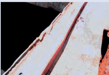
Mechanical damage to the compression bar and inner drain channel.
