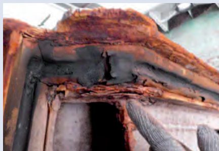
Hatch cover sealing rubbers damaged and showing permanent deformation beyond the recommended limits. Rubber seal channels severely corroded.
