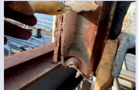
Hatch cover sealing rubbers damaged and showing permanent deformation beyond the recommended limits. Rubber seal channels severely corroded.
