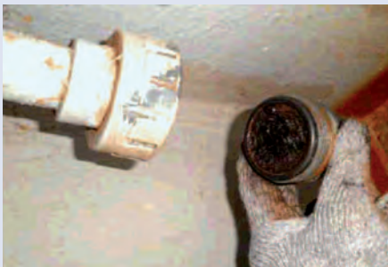
Hatch coaming drain completely blocked with debris and rust.
