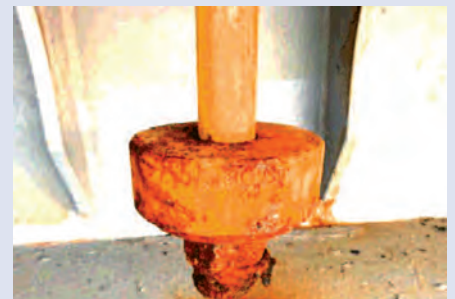
Hatch securing cleat, seized and painted over.
