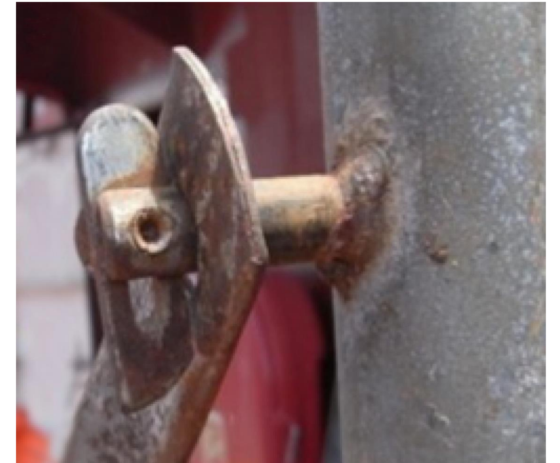
Loose scaffolding cross brace locking pins
