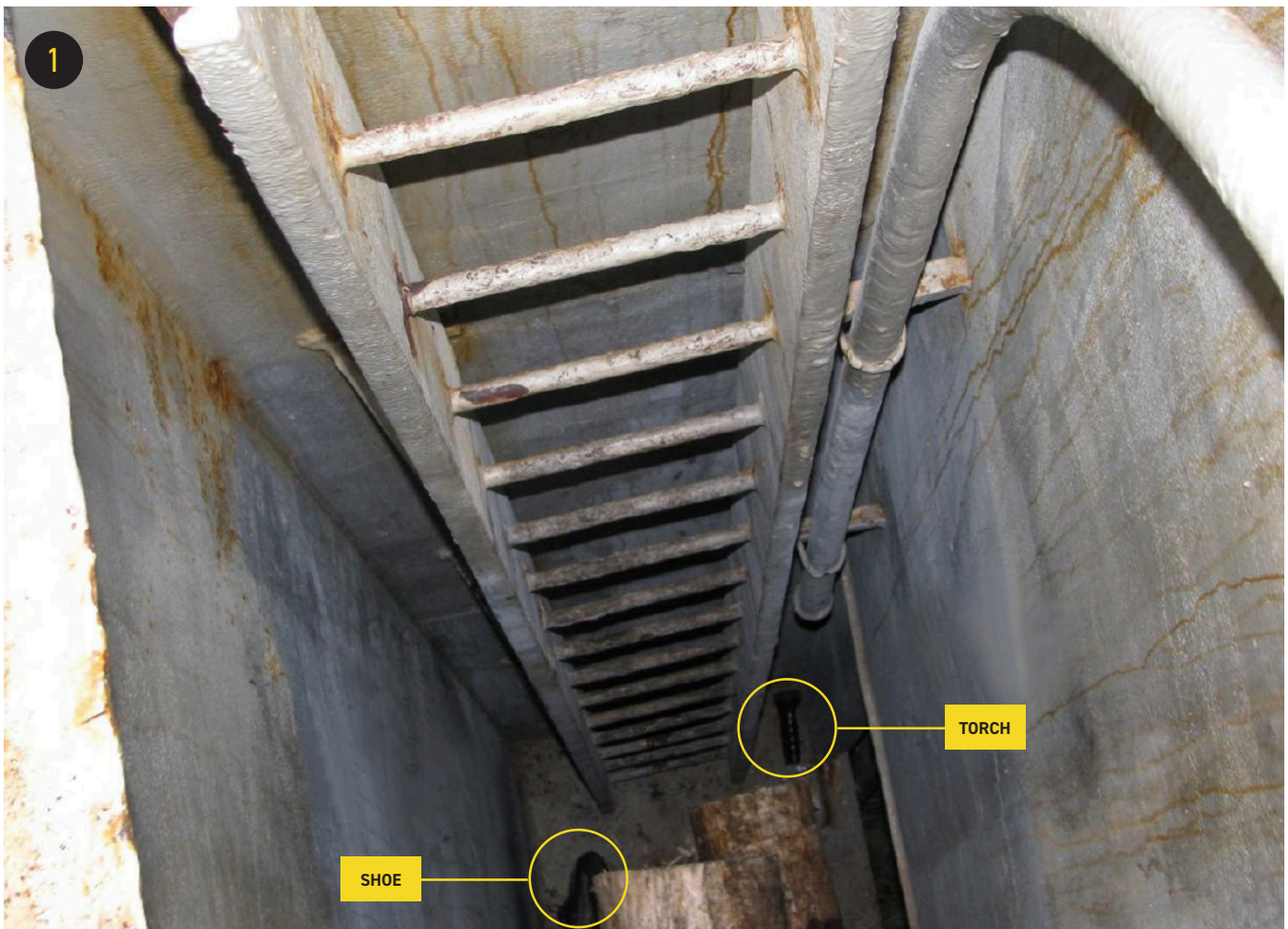
FIGURE 1 NO.5 HOLD AFT ACCESS SHOWING SHOE AND TORCH UNABLE TO BE RECOVERED SOURCE INVESTIGATION REPORT BY THE TRANSPORT ACCIDENT INVESTIGATION COMMISSION, NEW ZEALAND
