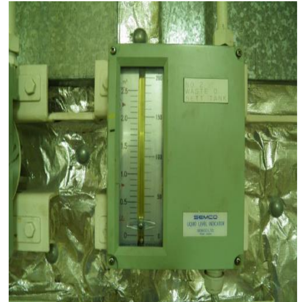
The malfunctioning level gauge
