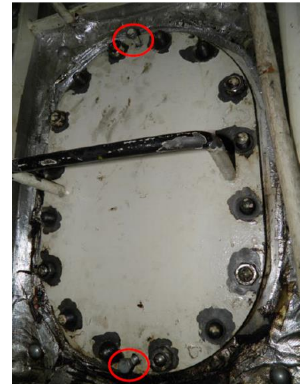
The manhole cover of the tank and the two jackscrews fitted on the top and bottom side.
