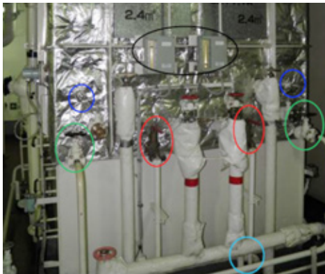
FIGURE 2 THE TWO WASTE OIL SETTLING TANKS. BLUE: THERMOMETER GREEN: DRAIN TO BSO TANK RED: SELF-CLOSING VALVE LIGHT BLUE: SCUPPER BLACK: LEVEL GAUGES SOURCE: HBMC I
