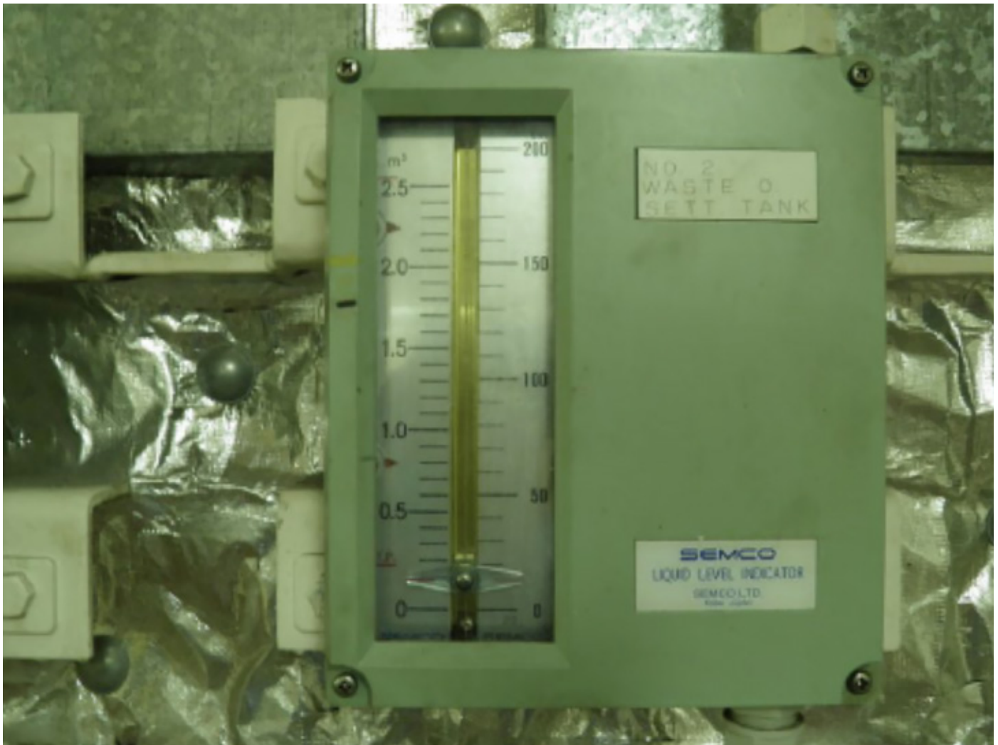
FIGURE 1 THE LEVEL GAUGE OF NO.2 WASTE OIL SETTLING TANK. SOURCE: HBMCI
